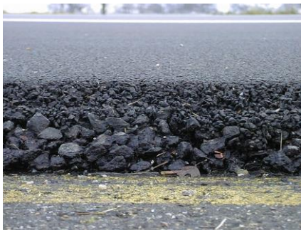
Figure 7: Double layer porous asphalt has a top layer, 15 – 30 mm thick, with small stones ( \leq 8 mm), and a bottom layer, 30 – 60 mm thick, with larger stones ( \leq 16 mm)
